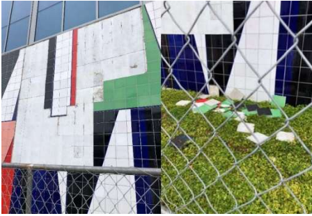
Damage to the walls of the Miami Beach Convention Center (photo courtesy of Miami-Dade County Courts)
